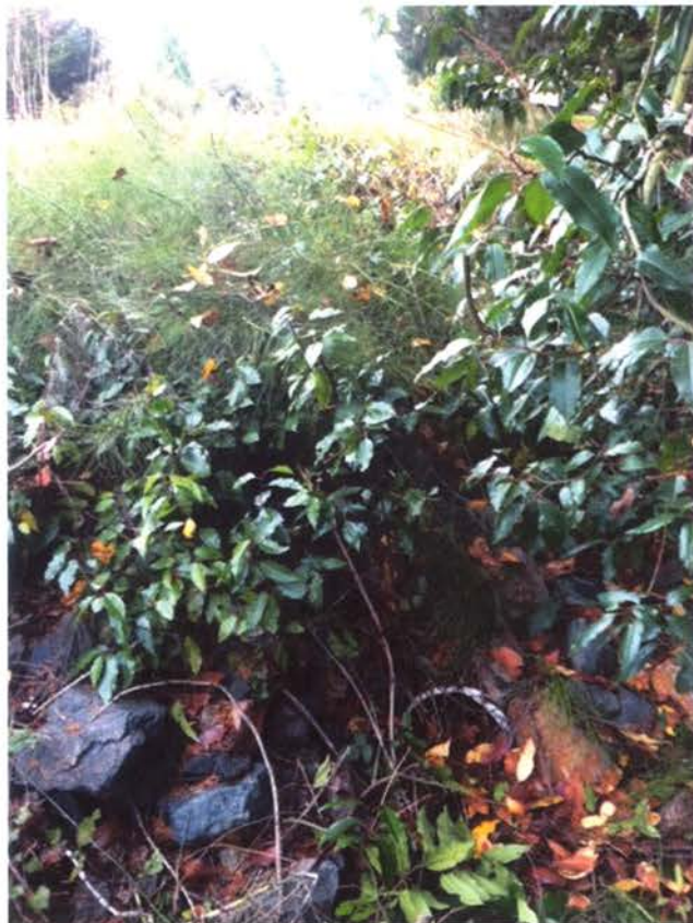
Photo H: Approximately 100 feet north of Photo G, looking south at 12-inch diameter corrugated metal pipe outlet and drainage ditch along the South (Betrozoff) Parcel.
