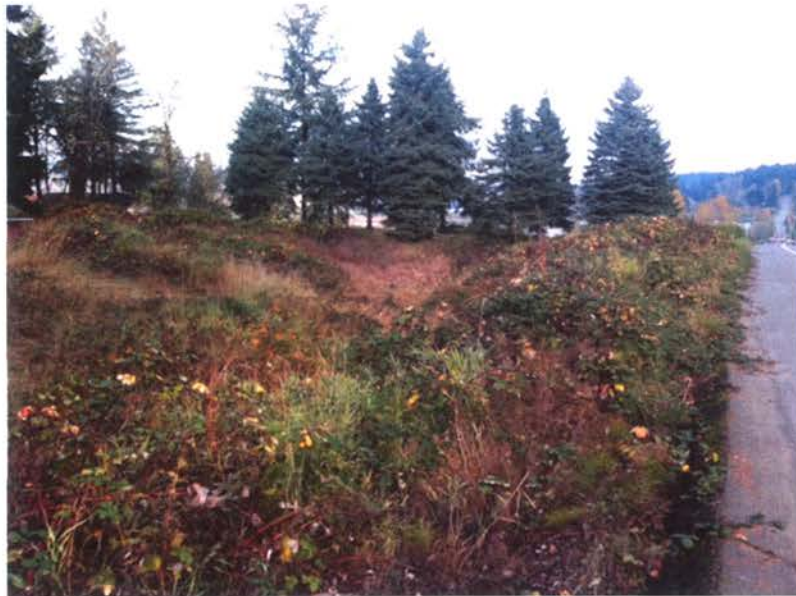
Photo D: Looking north at unmaintained roadside drainage ditch choked full of Himalayan blackberry and reed canarygrass. Drainage ditch located partly in public right-of-way and partly on the North (Jones) Parcel.
