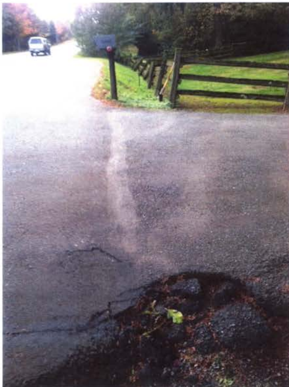
Photo B: Looking south at paved driveway entrance into the North (Jones) Parcel. Pavement is stained and showing watermarks from water overtopping pavement. 12-inch corrugated metal pipe outlet not found.
